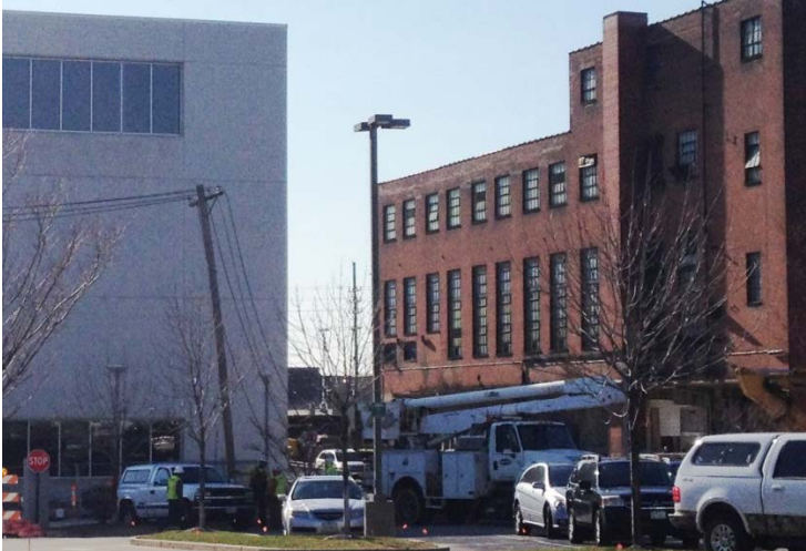
Utility wires and poles coming down along Duncan.
